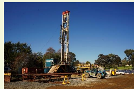
Geothermal production bore in Traralgon
